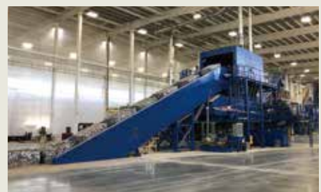
The Group's scrap melting furnace in the United States
