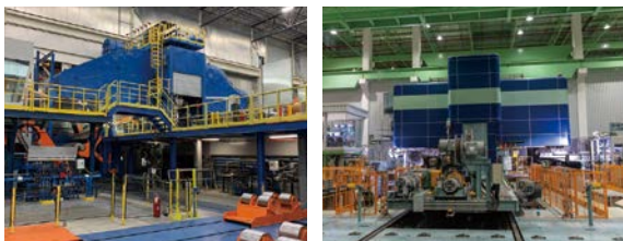
The newly added cold mill rolling lines at Tri-Arrows Aluminum (left) UACJ (Thailand)
