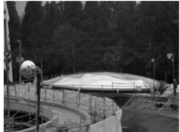
Fig. 6 Assembling of the Dome-Truss cover on the ground level beside the tank.
