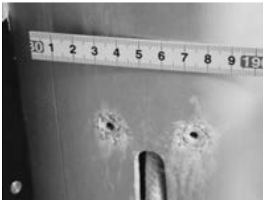
Fig. 6 Corrosion appearance of the screw circumference part of the cabin mast of the inside of "SUNTORY- Mermaid".
