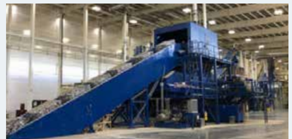
The recycling furnace began operating in 2018.
