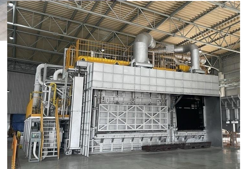
Side-well furnace Molten metal capacity: 120 tons (highest capacity in UACJ Group)
