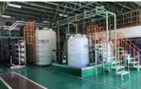
Water recycling equipment
