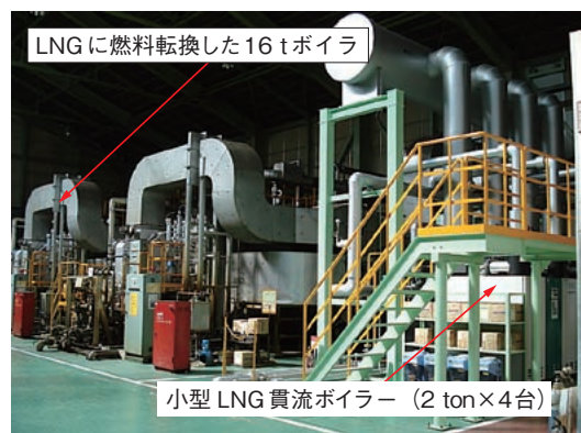
図10 ボイラ室全景 Fig.10 Full view of boiler room.
