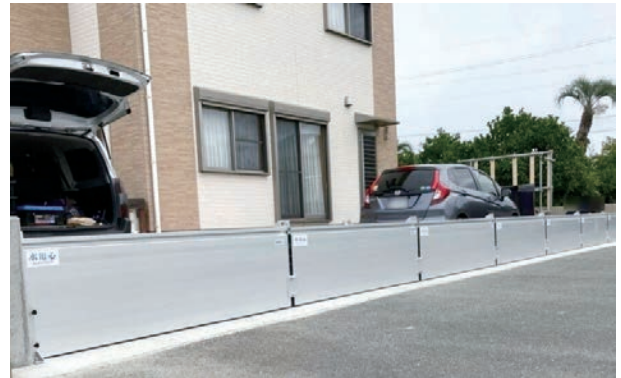
Fig. 6 Example of installation on a residential parking space with 14 meters width flood barriers.
